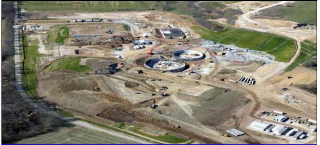
Aerial view of new Treatment Plant complex.
