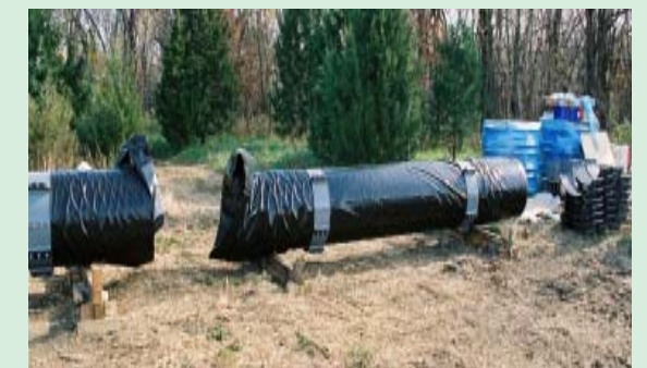
30" transmission main along K-7
