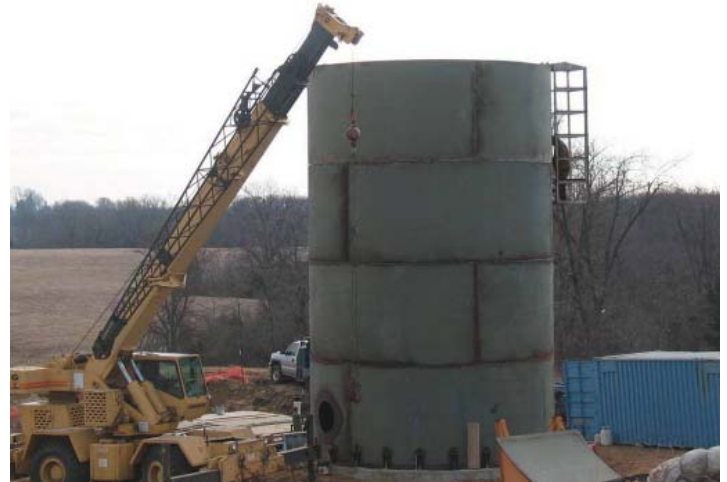
On-going construction of the 140-foot tall surge tank located near the Kansas Speedway.
