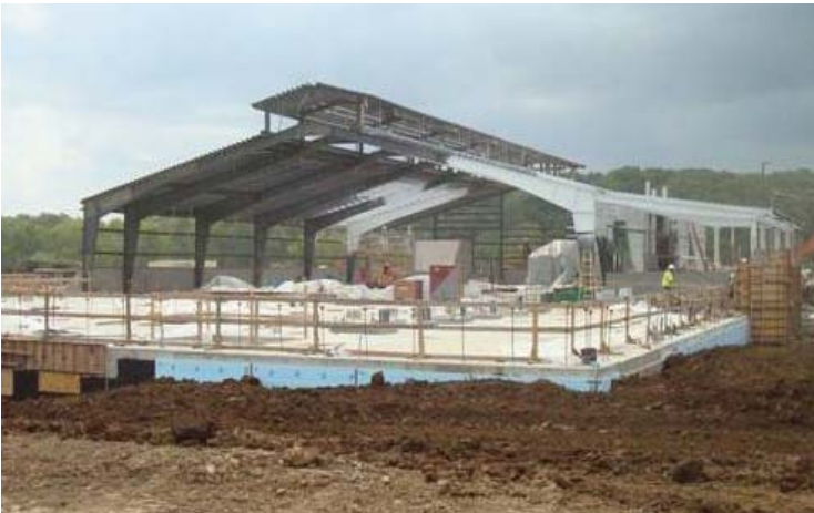
Operations Building located on Sam Clark Lane at the site of the new treatment facilities.
