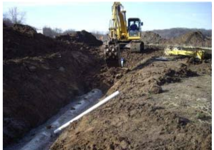
Photo showing pipe as it looks when installed.
